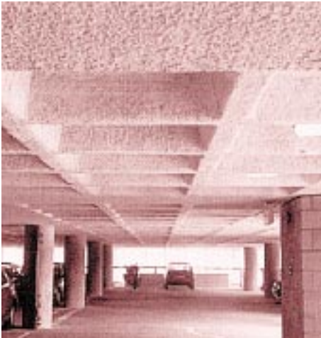
Spraydon TI applied for thermal insulation and fire protection to a basement carpark
